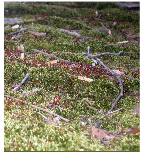
Top: fallen tree trunk. Photo by Colleen Crank. Middle and bottom: cabin roof and closeup of growth on cabin roof. Photos by Eddie Jones.
