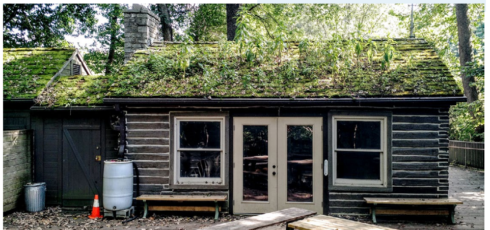
The Cabin roof overrun with fireweed, probably due to the wet summer. Photo by Eddie Jones.
