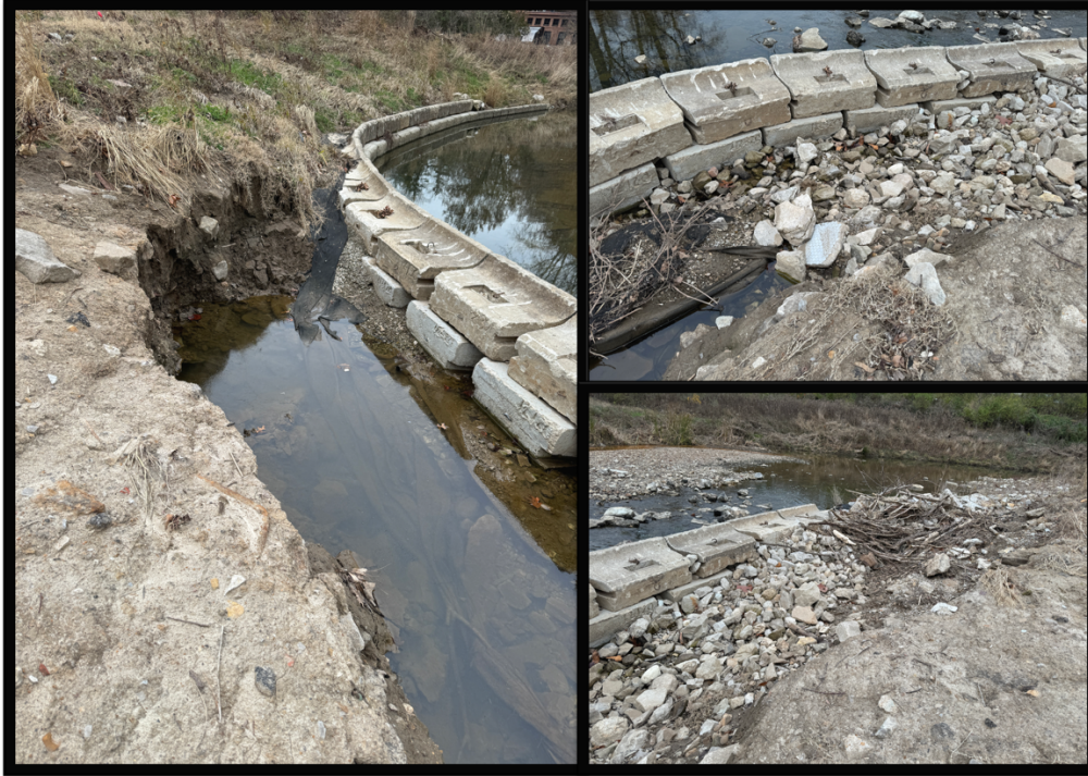
Figure 2. Severe scouring behind the toe wall on the banks of Deer Creek. Pictures taken on November 27, 2024.
